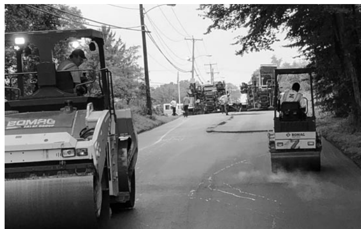
Road milling, paving and striping is underway throughout Monroe, thanks to the Township's $1.4 million capital investment, state grants and county infrastructure improvements.
