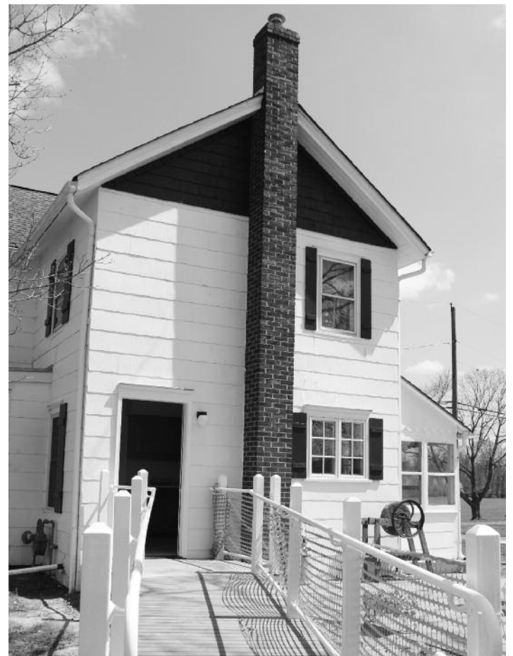
ADA upgrades are underway at the Dey Farm, which will allow physically-challenged visitors full access to the historic site's tours.
